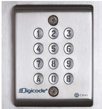
Figure 5.13 – Secure entrances can be accessed by authorized persons with their own code. 50
