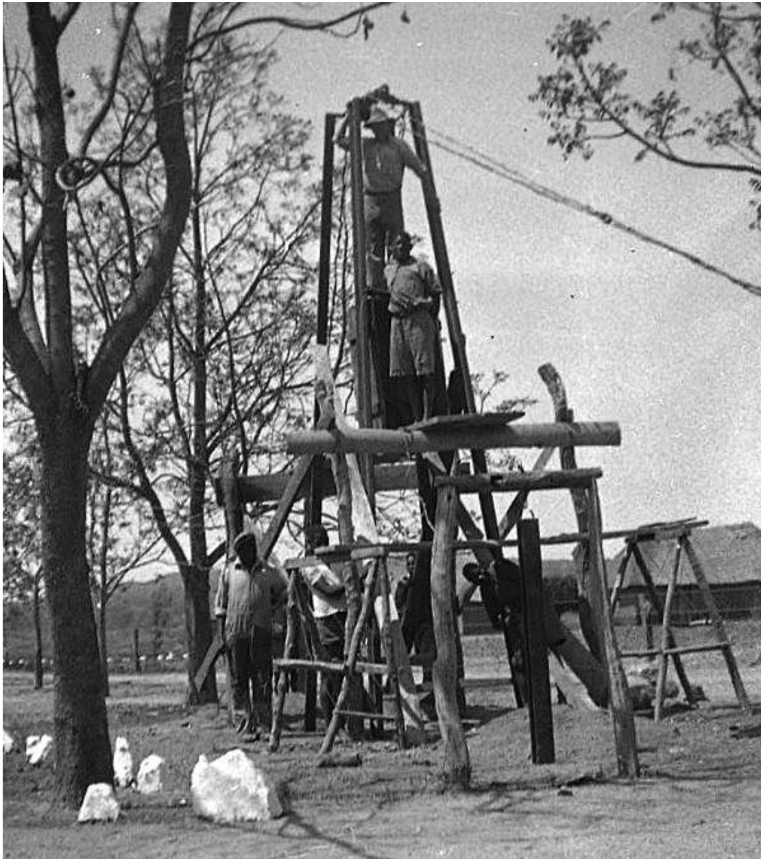
Myron Taylor Memorial Bell under construction. Photo courtesy of Cullen Photograph Collection.
